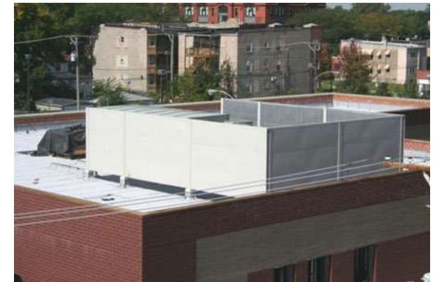
Figure 2-2: Roof Equipment Well Screened
