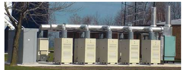
Figure 4-10: Biogas-Fired Microturbine Technology
