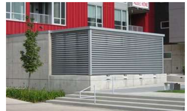
Figure 6-2: Appropriately Equipment Screened
