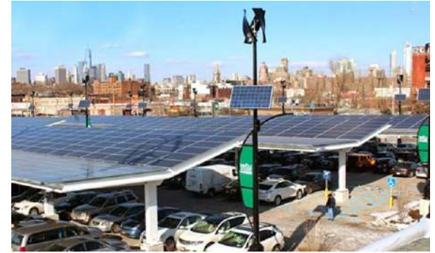
Figure 4-11: Solar Carports, Electric Vehicle Chargers, Wind Turbines and Solar Panels
