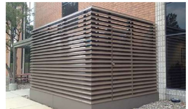
Figure 2-3: Side Equipment Well Screened
