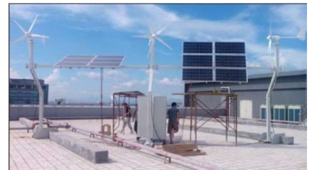
Figure 4-13: Rooftop Wind Turbine And Solar Panel Combination
